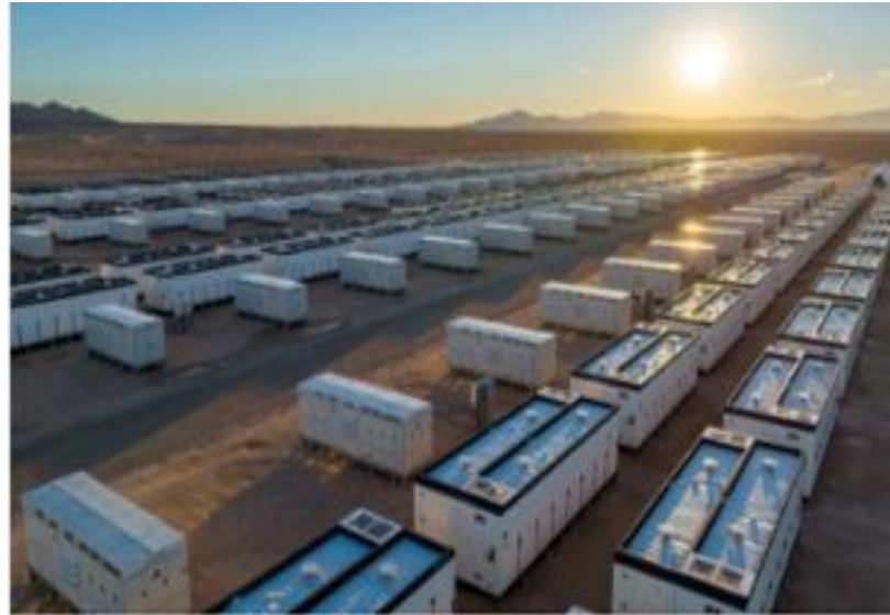
US PV+Storage 1.75GWh
