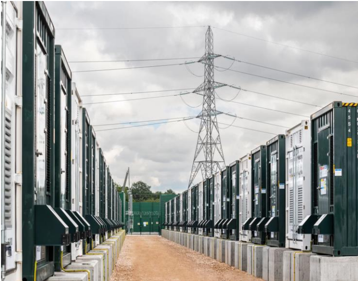
UK Reactive Power 100MWh
